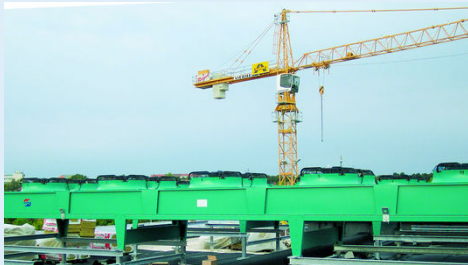
On the rooftop of the RPTC, there are 9 Güntneraxial drycoolers, model S-GFH 102C/2x5-S(D)-F4/2P.
