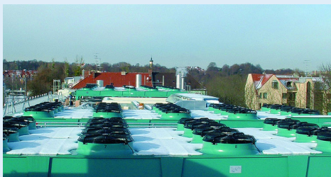
... to the mounting on the rooftop of the Rinecker Proton Therapy Center.
