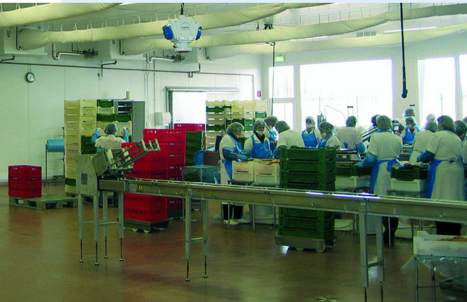
Air cooler with connected textile air socks for draft-free air distribution in the processing room
